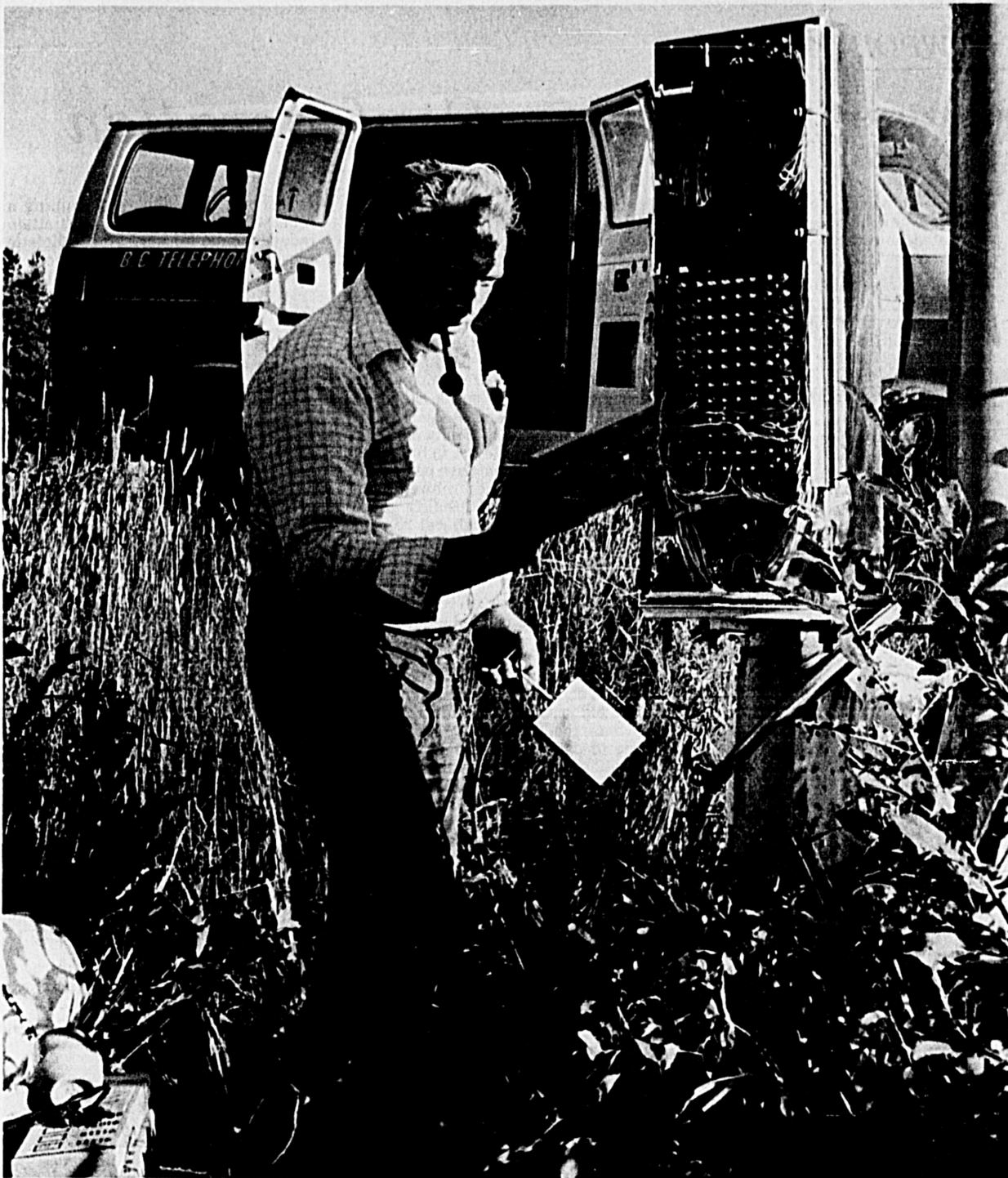
George Forsythe tries to restore service to 963 numbers after backhoe tore cable Tuesday. Citizen photo by Jean Witte
