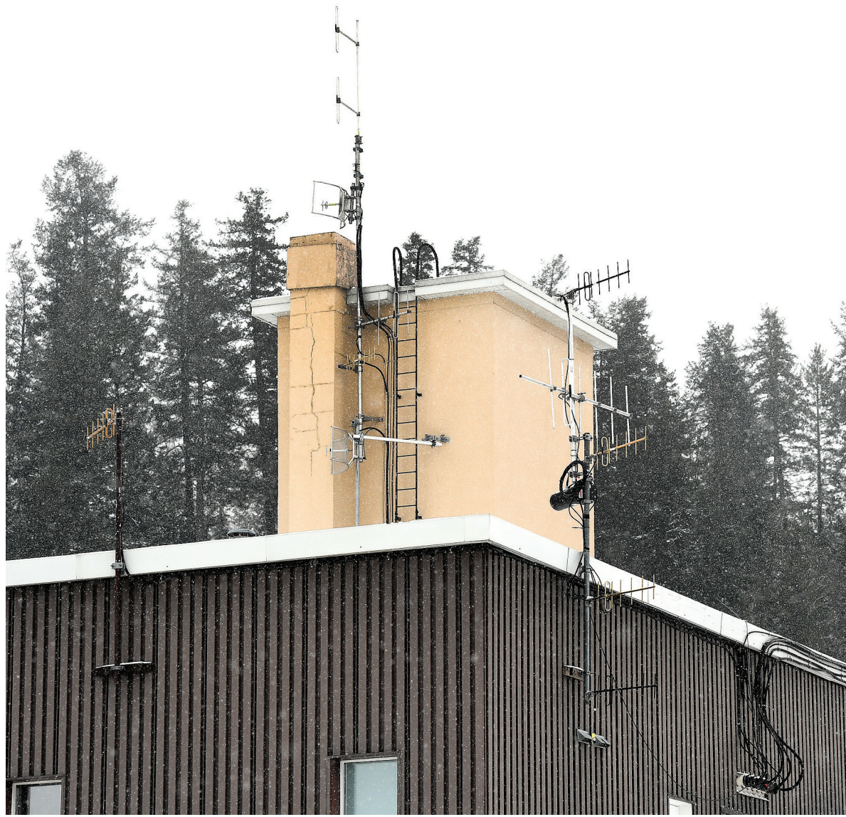
The antenna array on top of Fire Hall No. 1 is shown.
